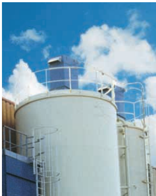
Jetline® E sur silo chaux Jetline® E on lime application
